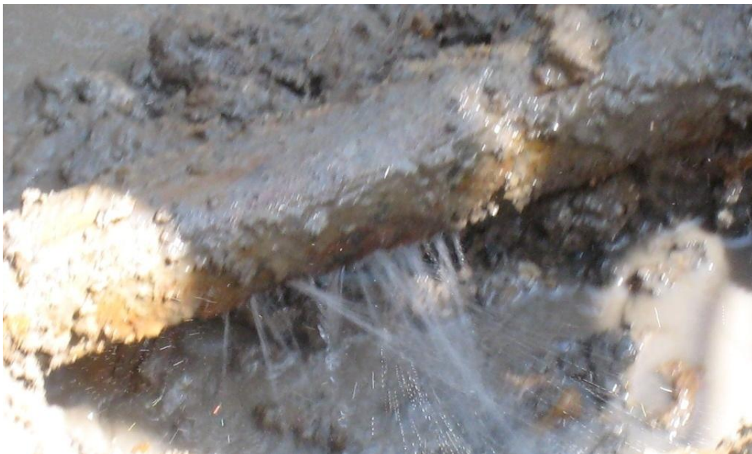
Figure 3. Longitudinal Crack 2” CI Pipe (325 W. 27 th Street)
