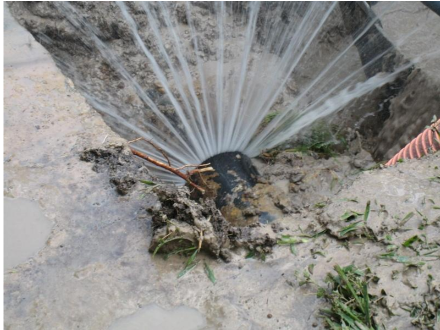
Figure 2. Circumferential Crack for 8” CI Pipe
