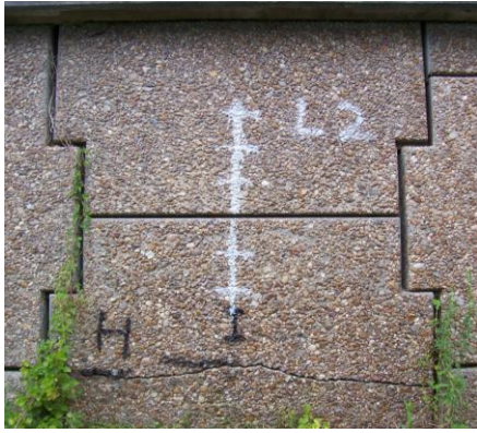
Fig. 1 Cracked panel in the retaining wall
