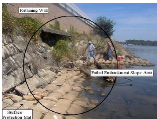
Fig.1. Embankment failure due to loss of fine particle by wave action
