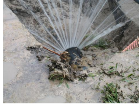
Figure 2 Full Circumferential Cracking
