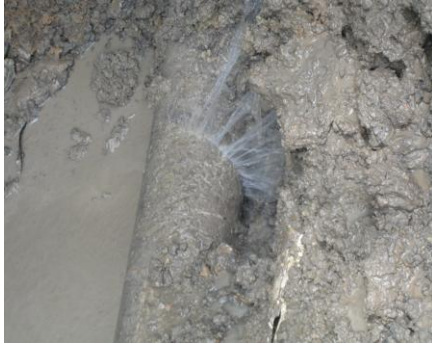
Figure 1 Partial Circumferential Cracking
